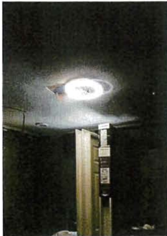
improper light, storage of new building materials
