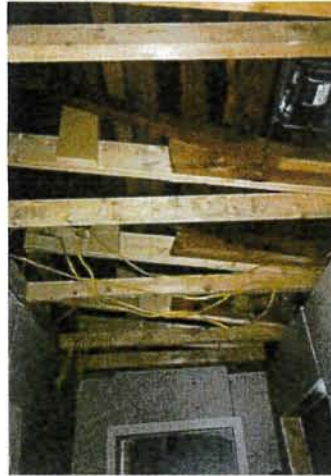
Exposed ceiling / no lighting
