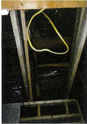
Exposed studs / wiring
