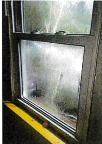
cloudy windows - not sealed.
