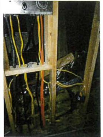
no wall between bathroom / storage, improper wiring
