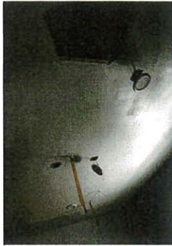
dangling light fixtures
