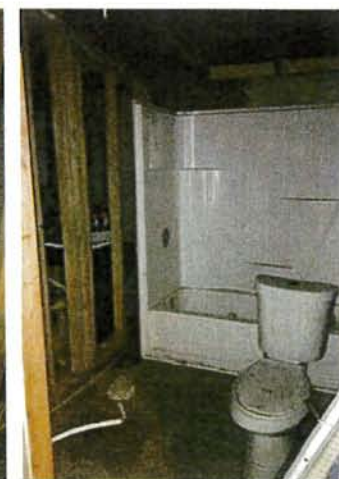
no bath fixtures connected
