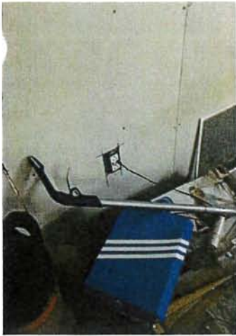
new unpermitted electric work
