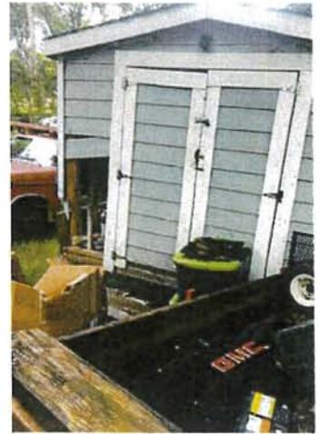
missing siding- accessory structure
