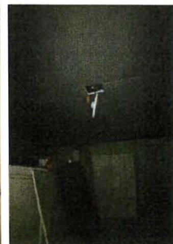
improper light mount
