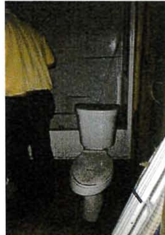
toilet not hooked up - only bathroom
