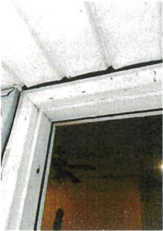
open air gap above front door
