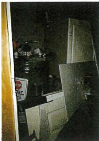
blocks & inoperable water heater
