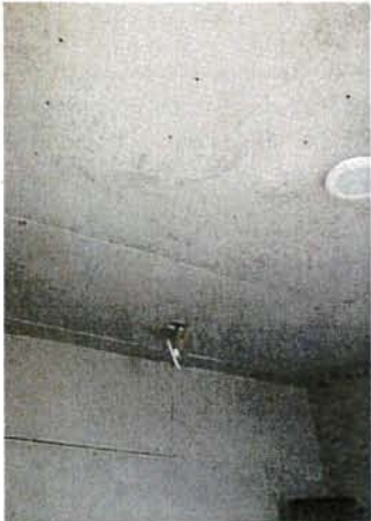
moisture spots on unpainted drywall
